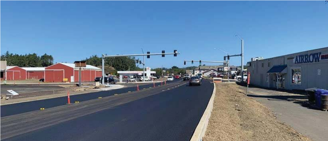
The new intersection of US 101 and SE 35 th Street that was installed as part of the 2021 US 101 improvements in South Beach creates an opportunity for redevelopment for adjacent parcels, including the Agency-owned site on the NE corner. Credit: City of Newport
